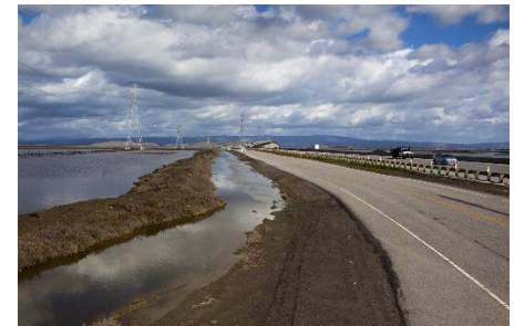
Water pooled near Dumbarton Bridge approach lanes.
