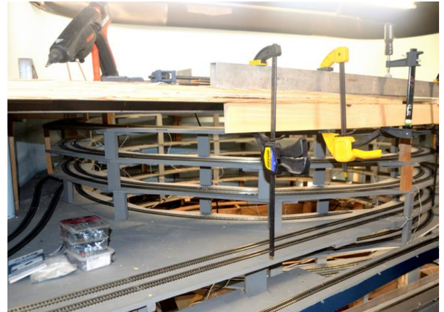
Above: This photo shows the progress of the helix construction on the new layout of the Garden State Railway Club in North Haledon.
