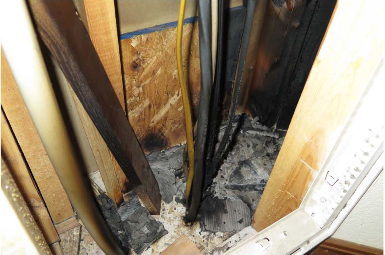
Figure 2. Burned corrugated cardboard in plenum/chase behind the air return grate.
