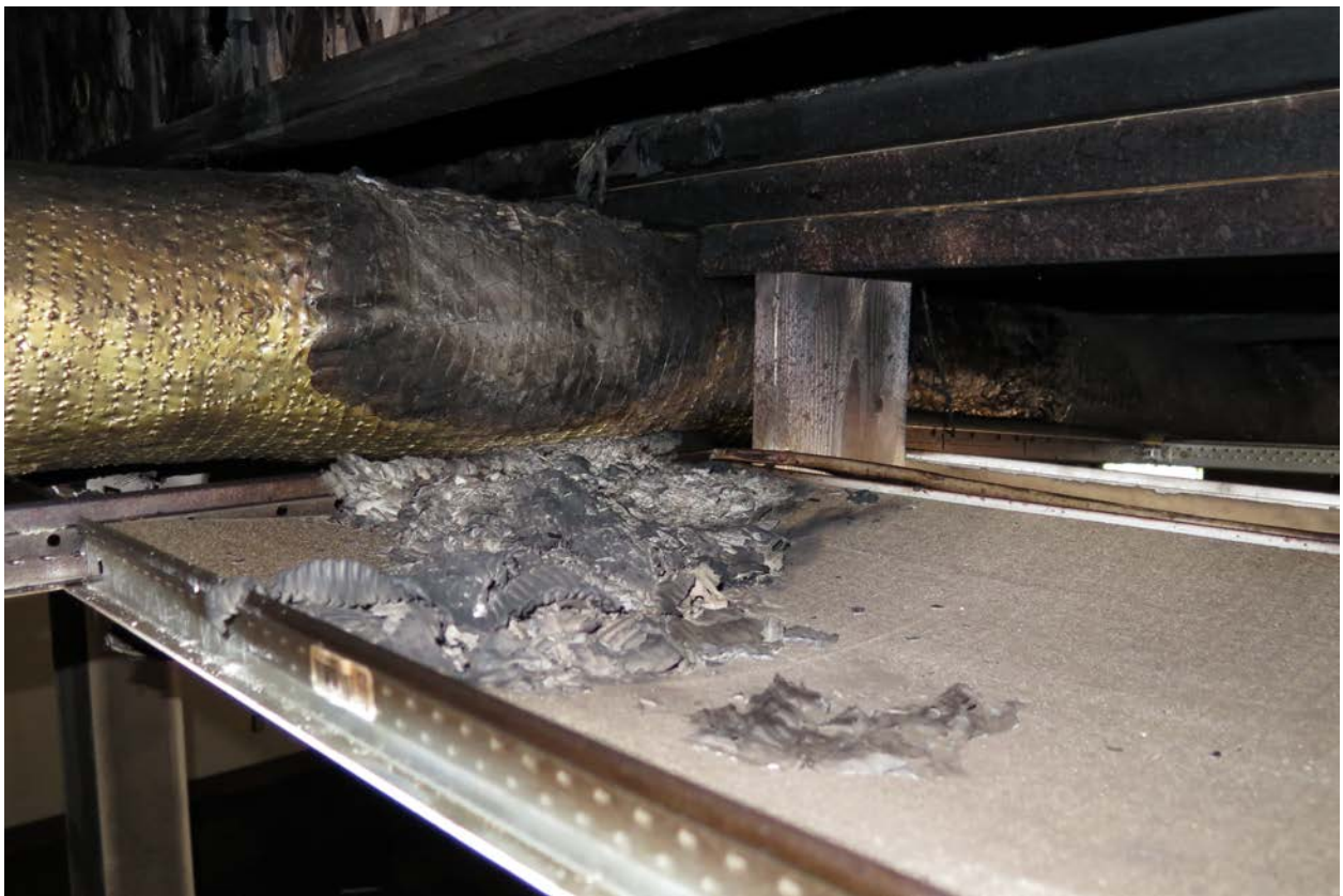
Figure 3. Burned corrugated cardboard found above the basement ceiling.
