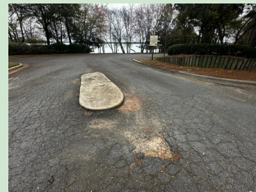
Photo on the right is the old entryway-- notice the cracked and worn asphalt.
