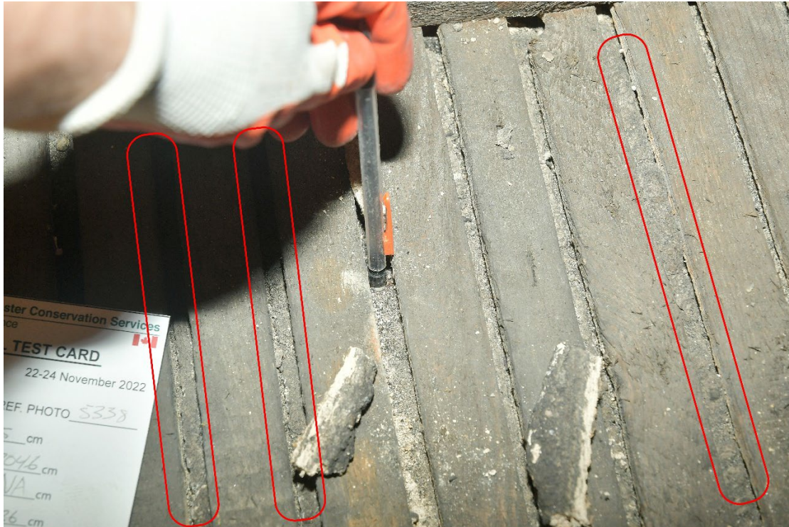
Figure 13: An area where the plaster is separating from the lath. Non-viable keys that have slipped through the lath spacing are circled in red. These keys did not break. (Three keys not circled were properly formed but had broken.)
