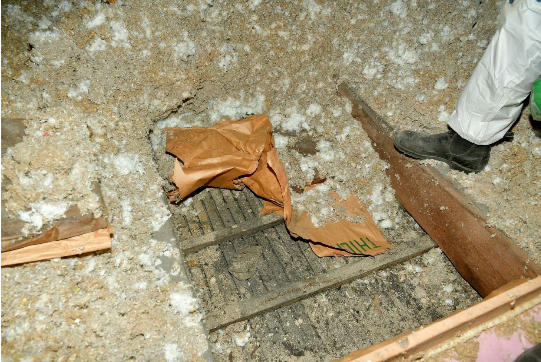
Figure 4: A partially cleared inspection location. The loose fill cellulose insulation covers a layer of rock-wool paper backed batts (removed in this image). The loose fill covers the top of the joists. Strapping runs perpendicular to the joists and is at roughly 30cm intervals. Note the near total lack of keys at this location even before testing (Location 3).
