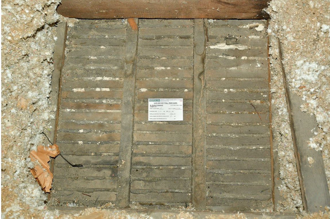
Figure 8: A test location after the insulation was removed and the area vacuumed. (Location 2).
