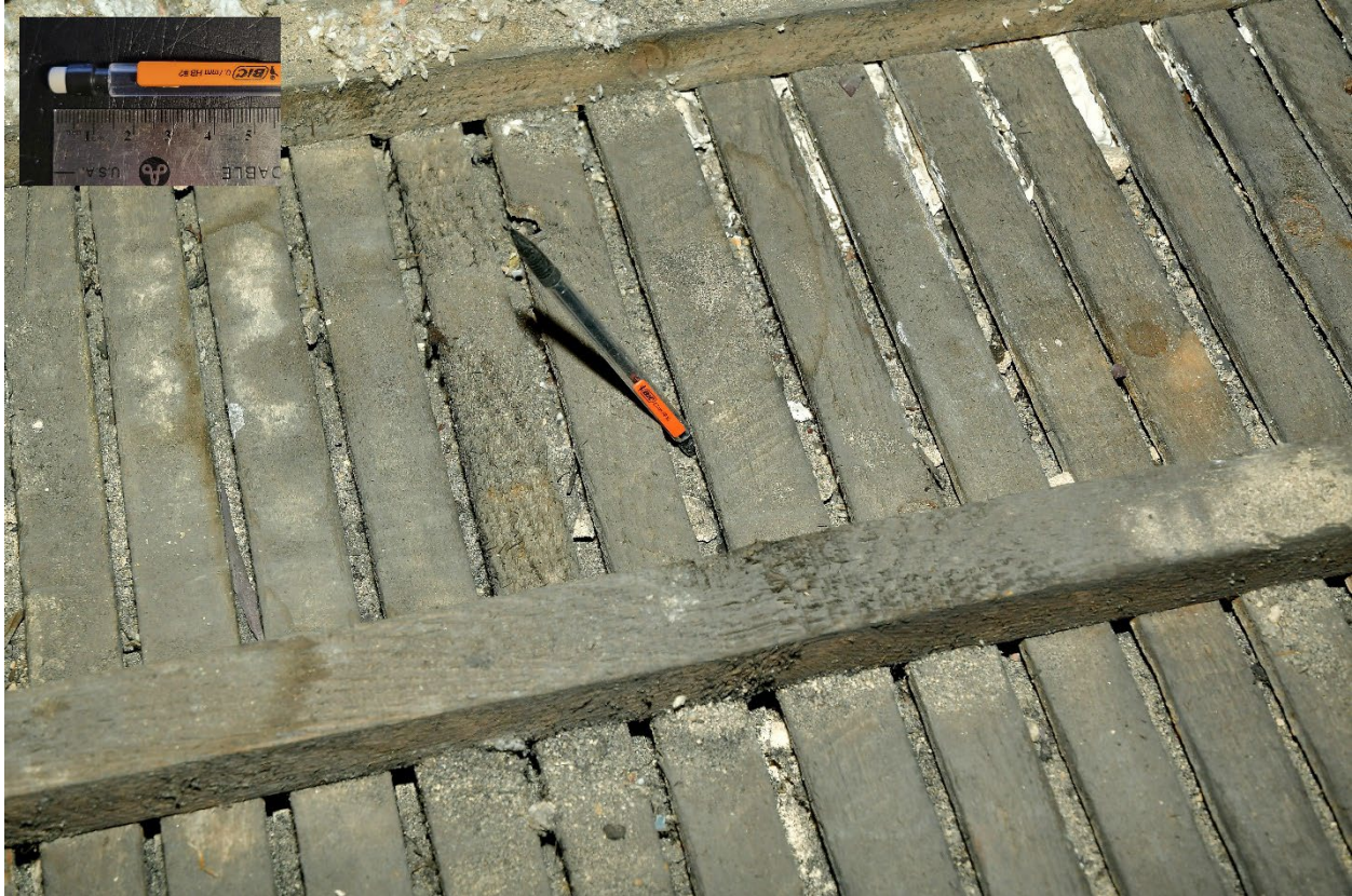
Figure 11. Plaster sagging away from the lath at test location 11. A similar condition was found at Location 2 and 3.
