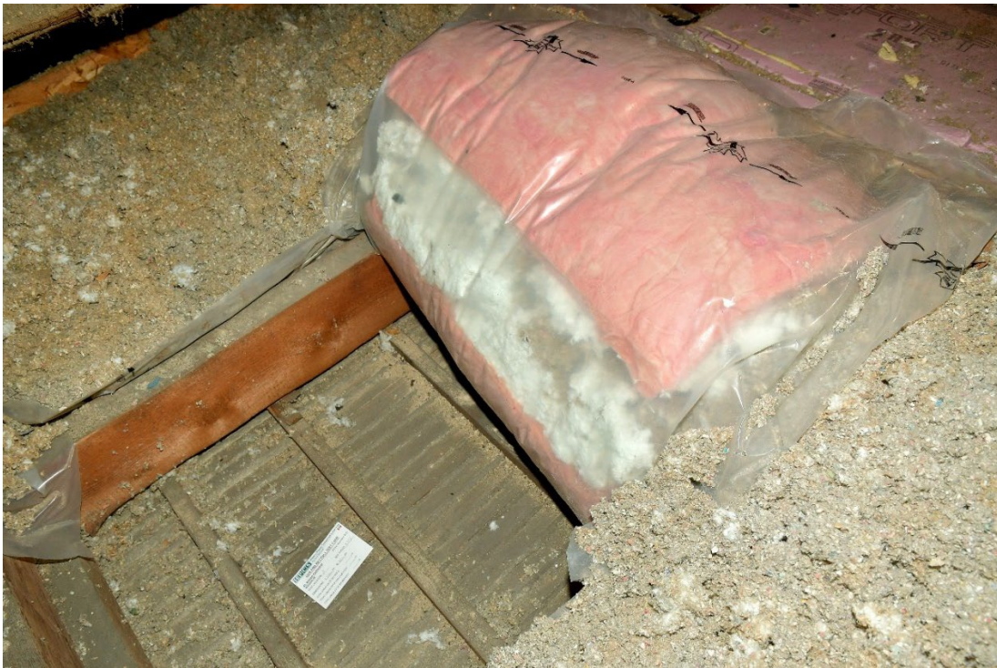
Figure 5: Newer insulation and a poly barrier were found at two of the test locations. The new insulation is hidden under the loose fill insulation so its extent is unknown.
