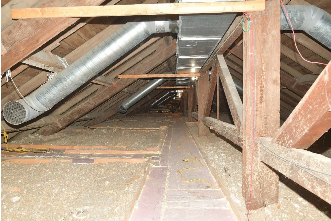
Figure 3: Attic conditions. Generally clean and well-kept. Mechanical systems are out of the way, and the catwalk is stable and secure.
