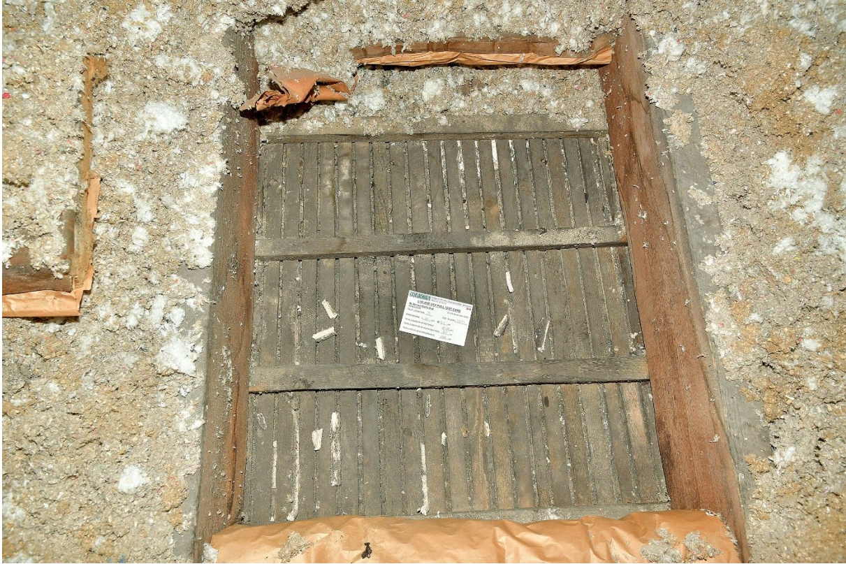
Figure 10: Near total key lost. Signs of water damage are clearly visible in the form of staining on wood (joists, strapping, and lath), and desiccated mold. There were many non-viable keys at this location, but it was difficult to count them as the plaster was sagging away from the lath enough to make it hard to distinguish old broken keys from non-viable.
