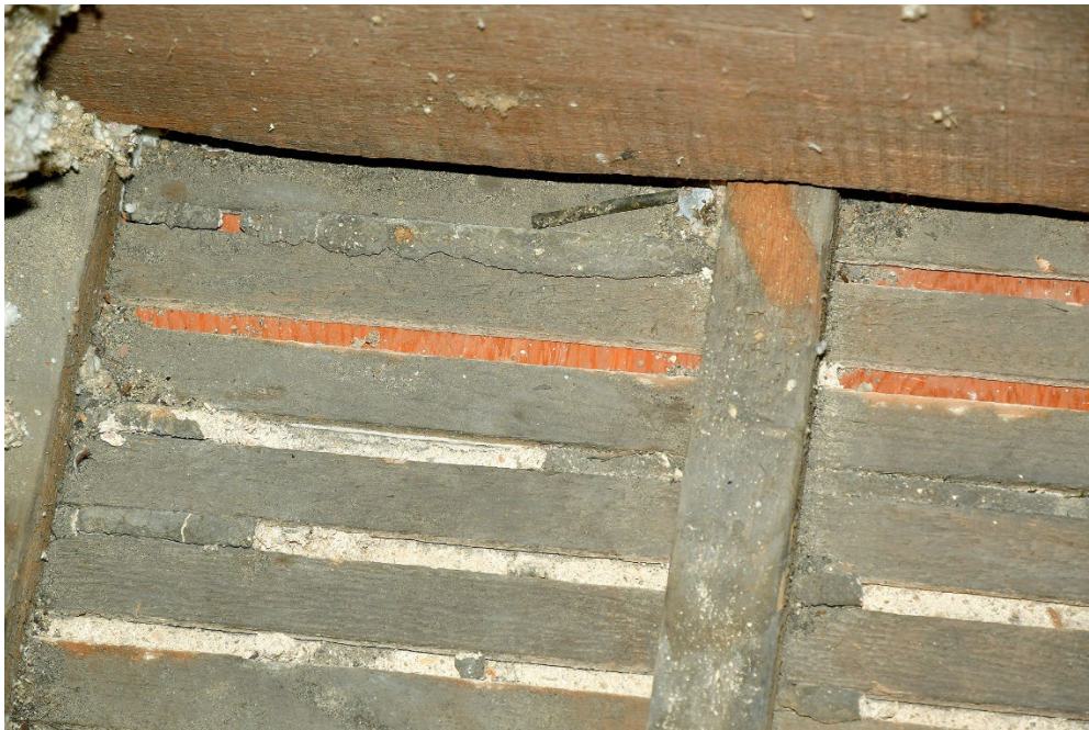
Figure 6: Plywood can be seen through the lath spacing at this location. The plywood is flush against the lath. The plaster near the plywood is in poor condition.
