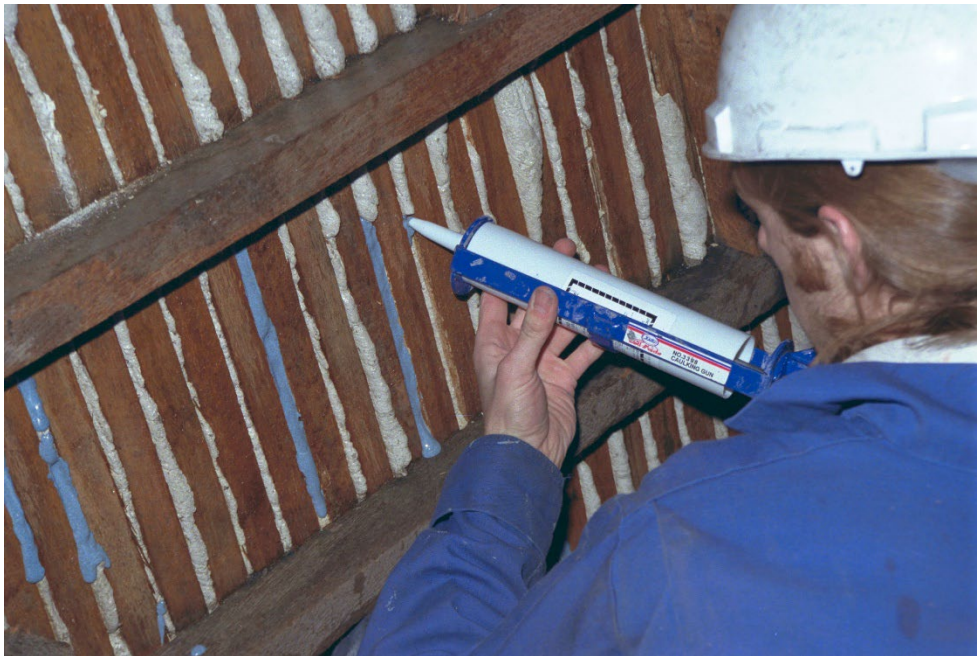
Figure 15: Missing lugs and keys are replaced with a lightweight, thickened variant of the consolidation agent.
