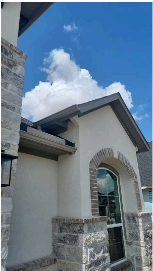
This missing kickout flashing was noted to the right of the front door when facing the property from the street.
