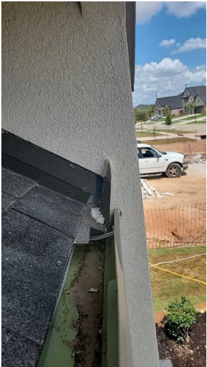
I observed an open or exposed penetration in the roof line at the time of the inspection. This was noted to the right of the front door when facing the property from the street. I recommend this open penetration is sealed to not allow water to get back behind the stucco veneer and cause damage behind the wall cavity.
