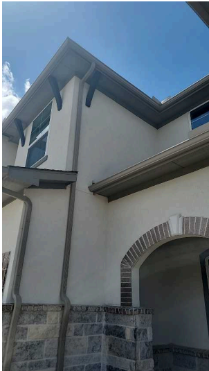
This missing kickout flashing was noted between the garage and the front door.
