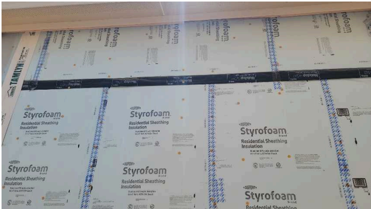
I observed the sheathing insulation was not butted up so that the top section is not flush with the lower level and creating a potential area for water leach down into the wall. This was noted on the right of the front of the home when facing the house from the street.
