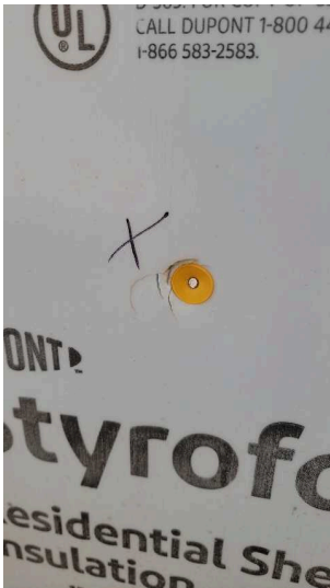
This was noted on the left side of the house when facing the property from the backyard.
