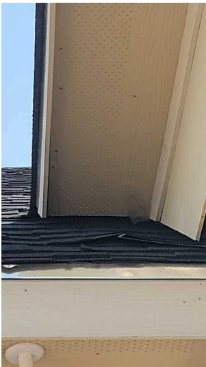
I observed flashing needed to be reset on the roof covering material at the time of the inspection. This was noted on the left side of the back porch over the AC secondary condensate lines.
