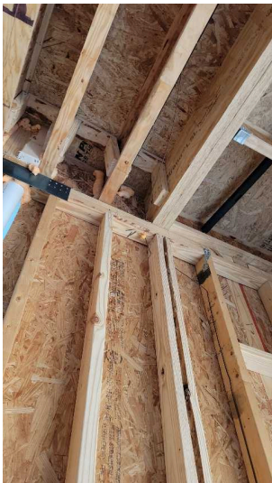
I observed missing fire caulk at the time of the inspection. This was noted in the garage in the stud bay above the double top plate.
