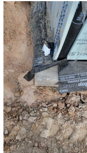
This was noted throughout the perimeter of the home.
