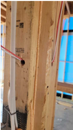
This was noted in the laundry room on the wall near the garage entrance.
