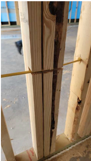
These missing nail plates were noted in the front room next to the garage.
