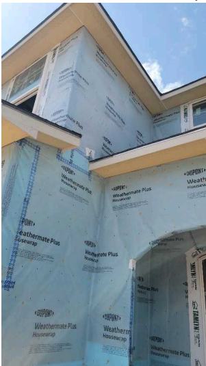
This was area lacking kickout flashing was noted over the front porch.
