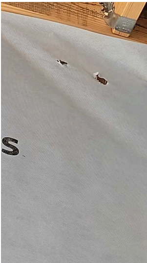
This was noted on the top left near the front door area.
