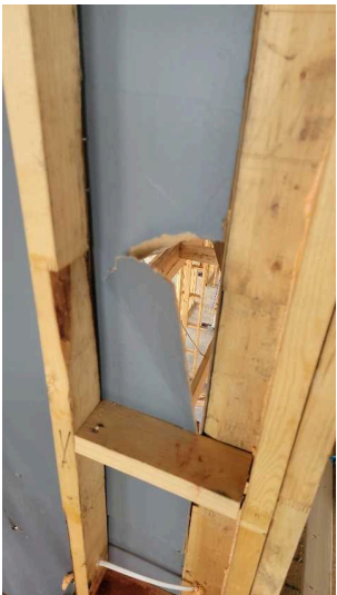
I observed a tear or puncture in the structural sheathing. This was noted in the upstairs wall in front of the top of the staircase.
