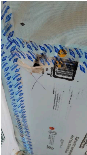
This was noted near the front door on the right.
