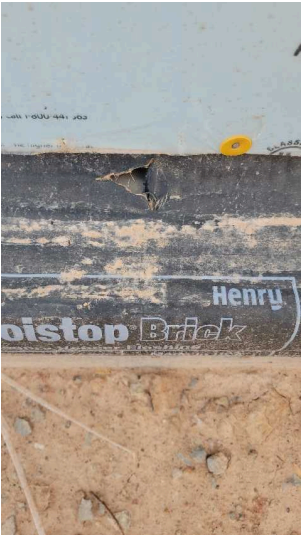
This was noted throughout the perimeter of the home.
