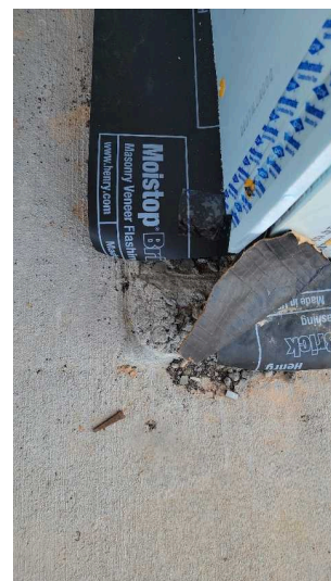
This was noted throughout the perimeter of the foundation wall.
