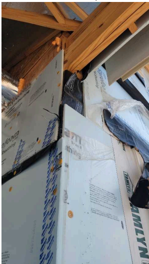
I observed a section of the exterior wall to be missing structural sheathing at the time of the inspection. This was noted to the right of the back porch.
