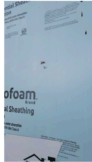
I observed a fastener was driven through the housewrap at the time of the inspection. I recommend it is sealed with flashing tape as holes, tears and other types of damage can potentially reduce its effectiveness. This was noted on the left side of the home above where the electrical connection point and meter will be.
