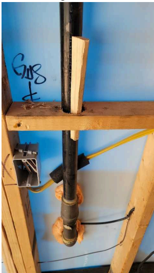
This missing nail plate was noted in the garage on the exterior wall.
