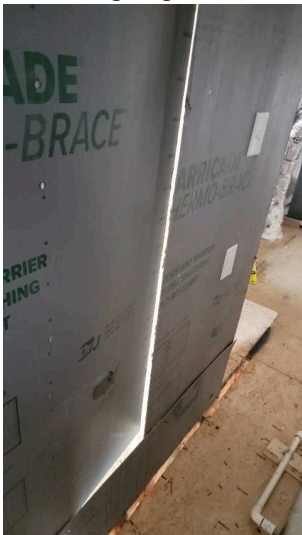
I observed the structural sheathing needed to be refastened. This was noted in the attic space.
