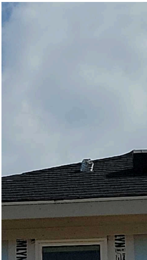
I observed an inappropriate vent material protruding through the roof at the time of the inspection.
