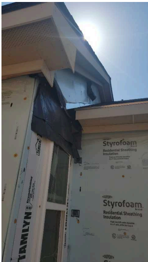
I observed kickout flashing to be lacking or needs to be extended further out. The kickout flashing details observed at the lower bottom edge of the roof line interface and the sidewall that continues past the edge of the roof should be extended if installed. Kickout flashing is installed to prevent water runoff from entering behind the exterior wall covering. The lack of a proper kickout flashing will allow water to penetrate at these points. This will also help to prevent discoloration of exterior walls at the bottom of the roof/wall intersection and direct water into the gutters. This was noted on the left side of the home when facing the property from the backyard.
