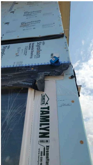
I observed tore masonry veneer flashing. This was noted over the back right window in the backyard on the right side.
