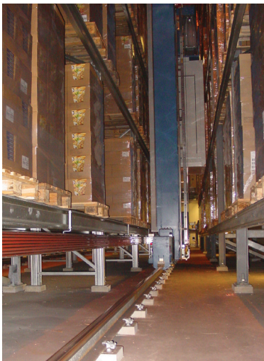
Feed and control for warehouse crane in deep freeze storage
