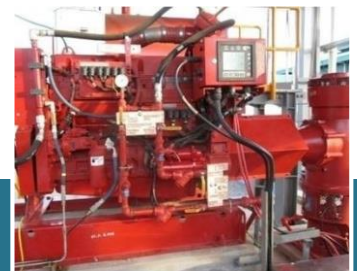
SOUTH SUMATRA NGL FAIRBANKS NIJHUIS; 2500GPM @2 UNIT
