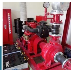
STASIUN KA CIREBON, 2019 FAIRBANKS NIJHUIS; CAP. 500GPM @110M, 2 UNIT,
