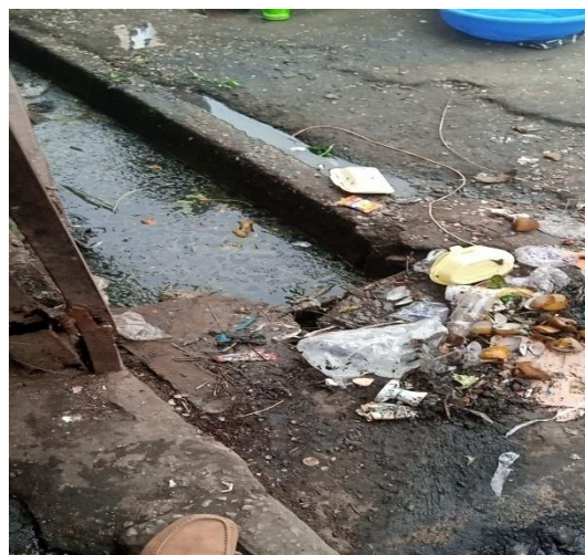
Plate 4: Blocked drainage/filthy environment at the leg of the pedestrian bridge at Watt Market
