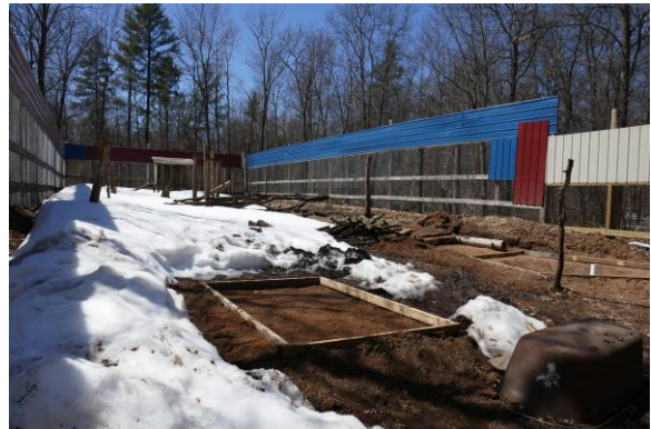
Yes, we shoveled snow so we could get our concrete frames done.
