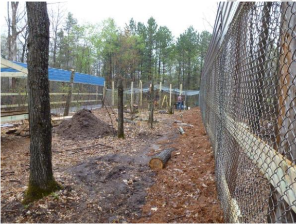
This is taken from the corner of the expansion looking towards Mark & Tim working on the wall between the old bear enclosure & the expansion.
