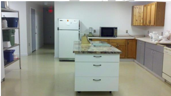
The kitchen island is finally finished. Now we just have to install the kitchen sink!
