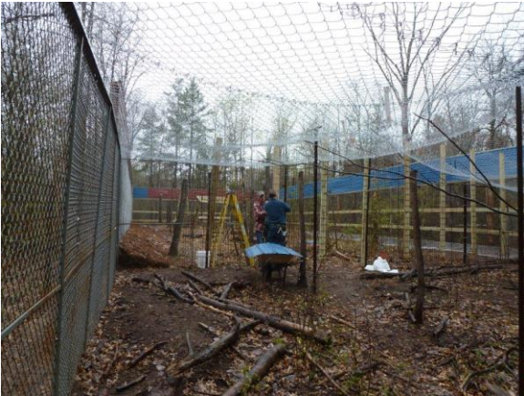
This is taken from the door of the current bear cage to show the expansion. Mark & volunteer Tim are working on preparing the wall between old enclosure and the new expansion.
