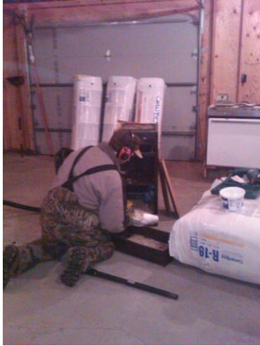
Insulating the garage...the only building on the property when it was purchased. Photo taken 2/8/11
