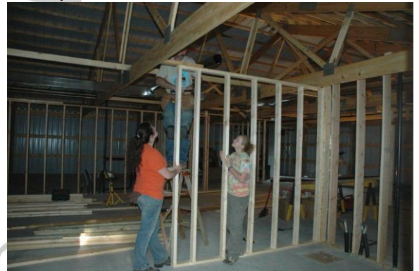
Heather, Mark and Kristina erect a wall on the dedicated cleaning room.
