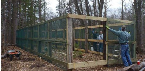
Volunteers Tim & Cheryl help install wire on the walls of another mammal enclosure.
