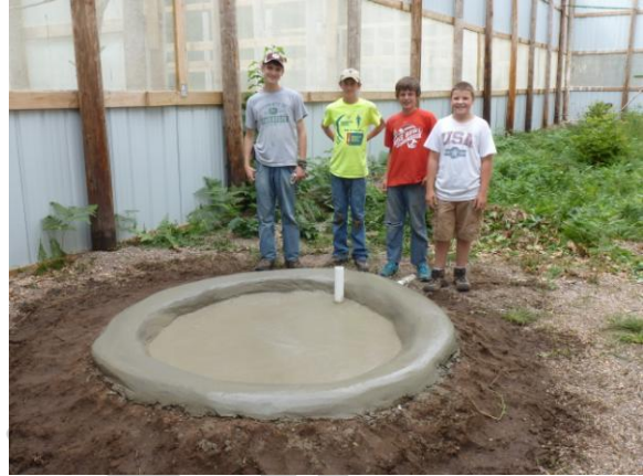
Marshall and his work crew show off the new eagle pond. All that's left to do is the gravel.
