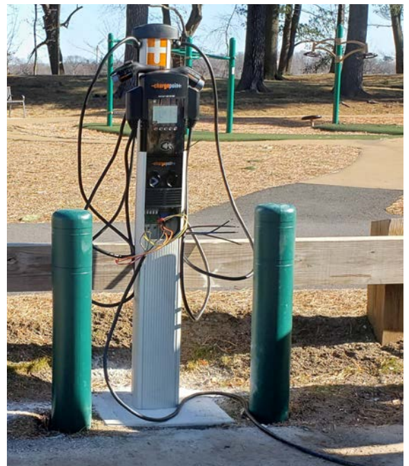
EV Charging Station at Farm Pond Park
