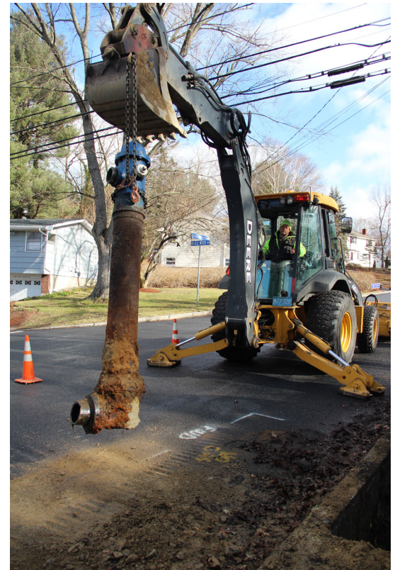
One of 51 hydrant replacements performed this year, this one on Old Worcester Road.
