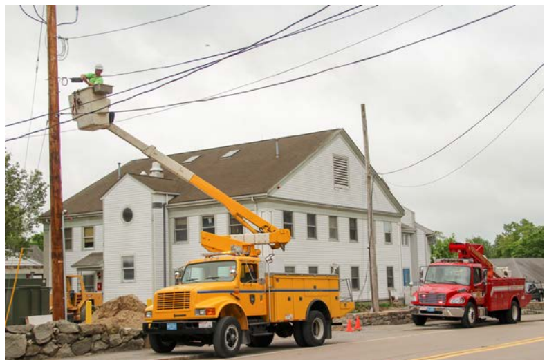
DPW staff installing some of the 3,355 feet of the new fire cable this year.
