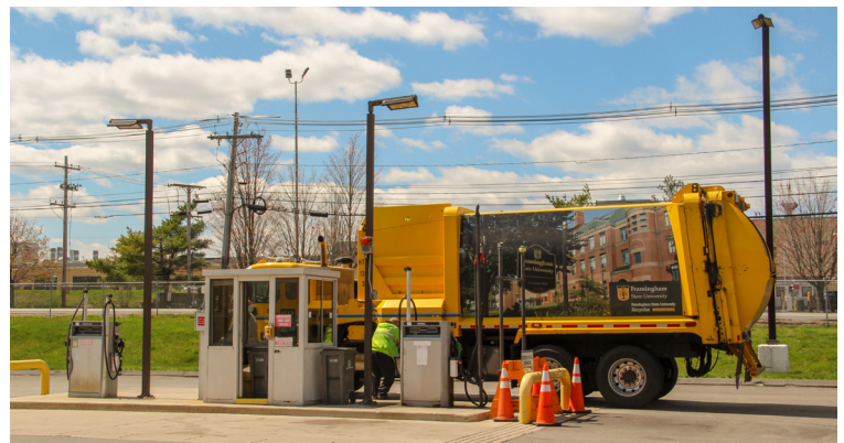
Fuel Island at the DPW Headquarters is utilized by numerous City departments.
