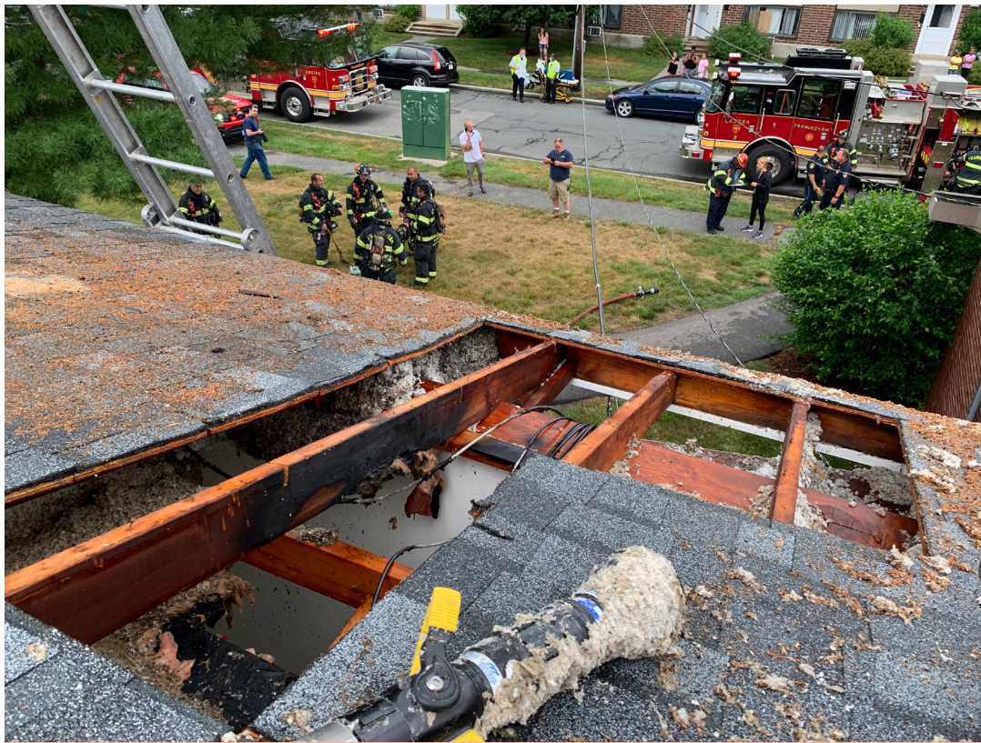
Structure fire extinguished
