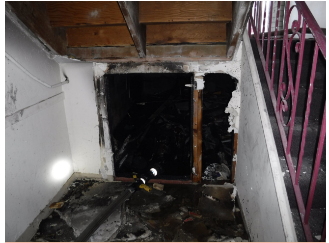
Exit foyer fire at 25 Willis Street
