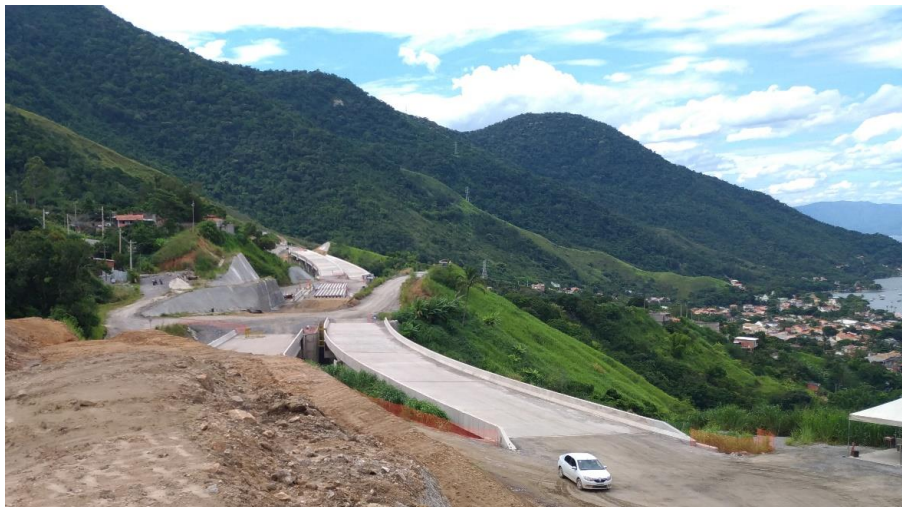
Figure 2. An example of a sector of the Tamoios Highway under construction. It is possible to see the Serra do Mar steep hillsides and São Sebastião urban area.
