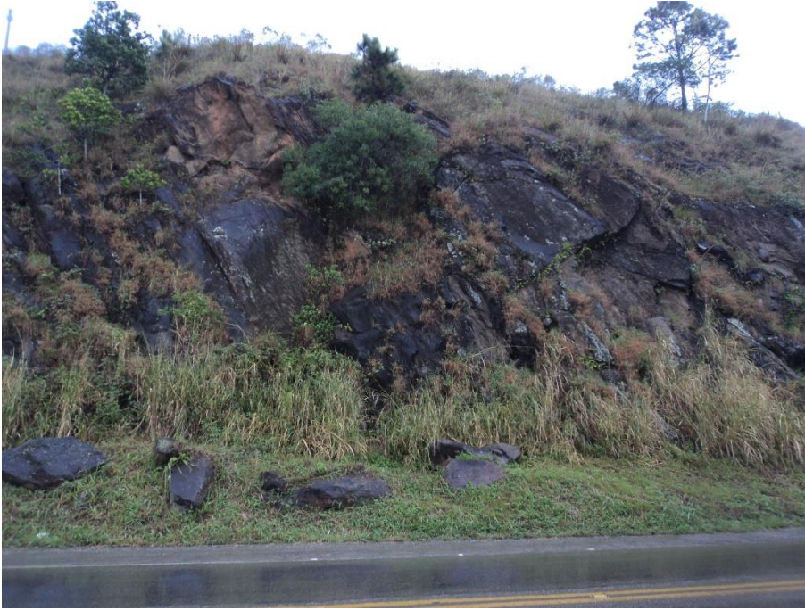
Figure 3. A slope at the beginning of the studied site. Notice the boulders at the slope's foot, and scars of failures in the rock slope, probably from rockfall events.
