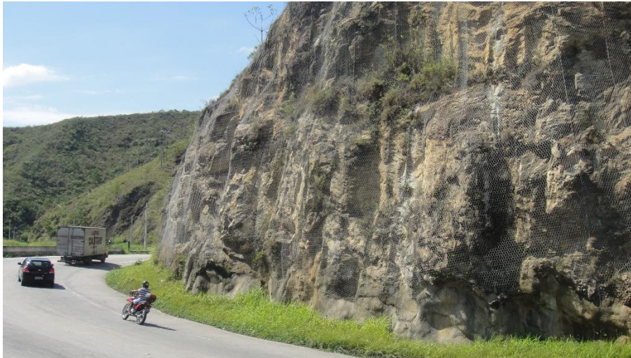
Figure 2. A slope just a few meters before the beginning of the studied sector. On this slope, there is already a metallic wire installed, with some rock boulders caught inside the net.
