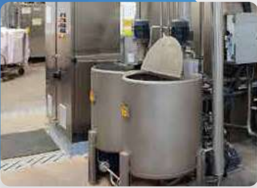
İLAVE TANKLAR ADDITIONAL TANKS
