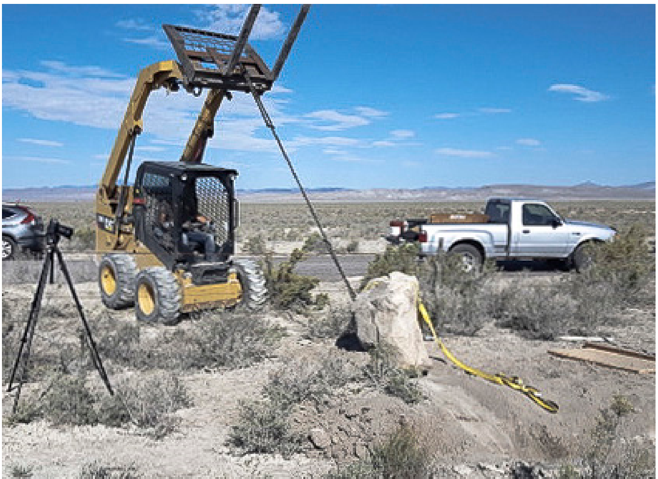
Forklift drags the James Wakasa memorial monument from newly-dug hole (at right) on July 27, 2021, Topaz, Utah. Dragging may cause damage to the artifact, especially if writing or carving had existed on surface. Photo courtesy Utah Division of State History.
