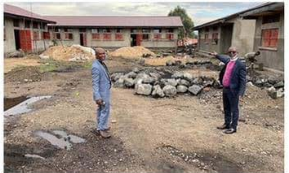
School facility under construction with a grant of $250,000.00 from the Government of DR Congo
