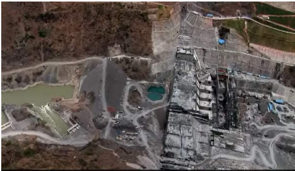
The Ahai Dam on the Great Bend of the Yangtze in northwestern Yunnan. The Liyuan Damsite. Photo by Adam Elliott, 2009
