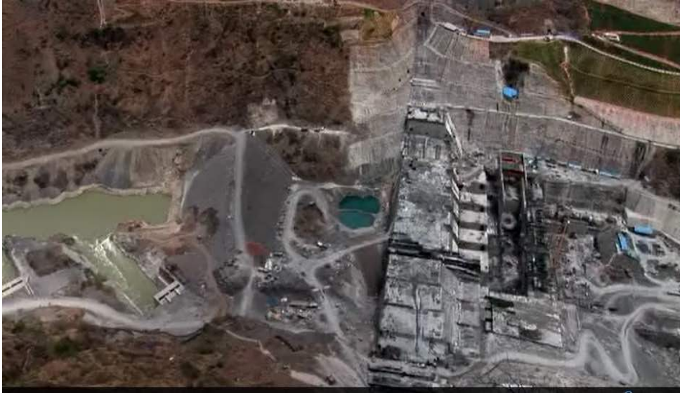
The Ahai Dam on the Great Bend of the Yangtze in northwestern Yunnan. The Liyuan Damsite. Photo by Adam Elliott, 2009
