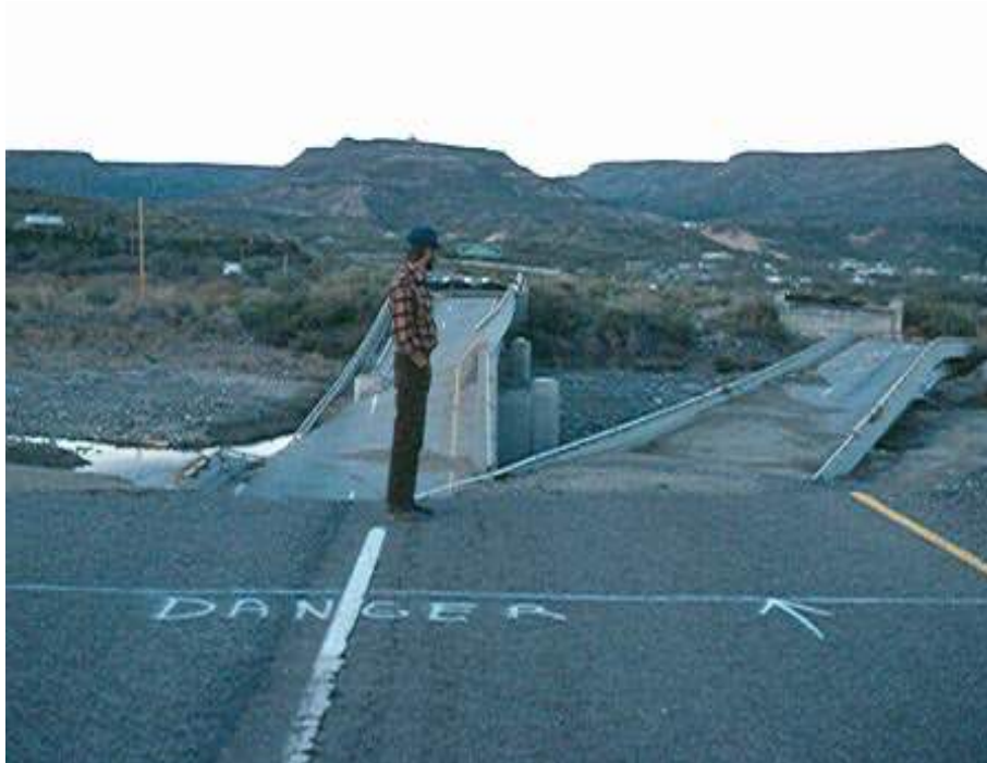
The author viewing what's left of the brand new I-17 bridge over the Aqua Fria after a hundred year flood in 1979. Photo by Cindy Appel.
