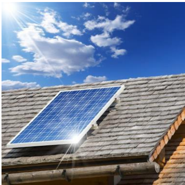
Solar panel on the roof
