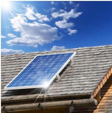
Solar panel on the roof
