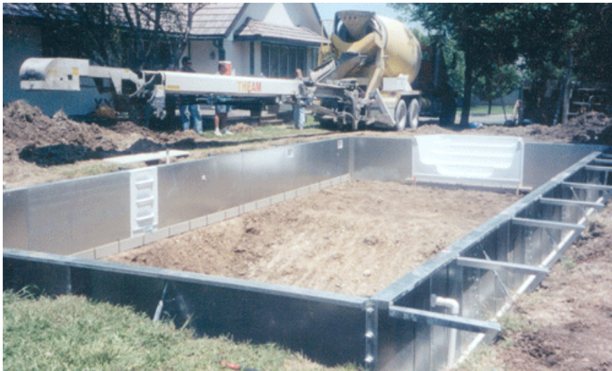
Photo B1 – Metal pool with fiberglass stairs and pool reinforcing brackets
