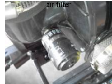
Dry-type air filter blockage alarm
