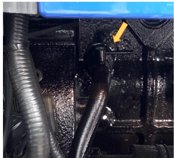
Water drain valve of cylinder
