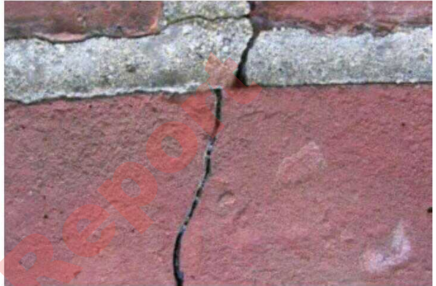
The bricks have split as well, showing that the base of the chimney is not properly supporting the chimney.
