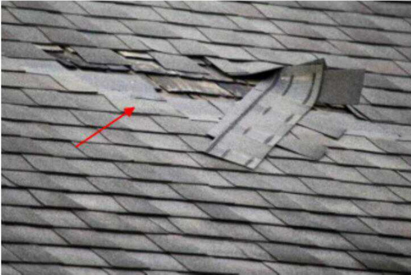
Tile are starting to pull away and there are leaks into the attic from this spot.
