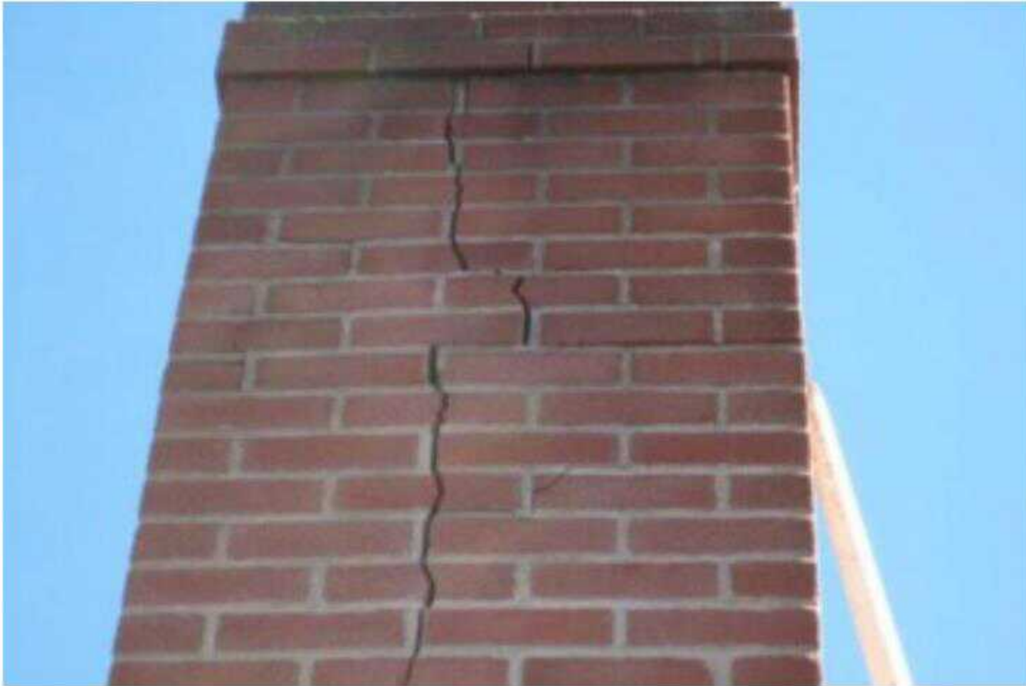
The chimney is cracked from the roof to the top of the chimney.
