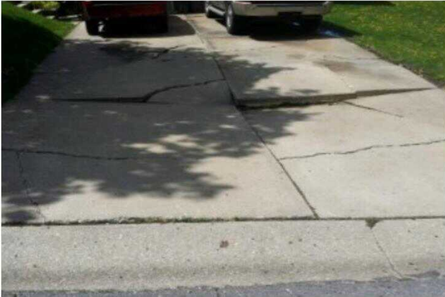
Cracks from the street all the way to the garage door.
