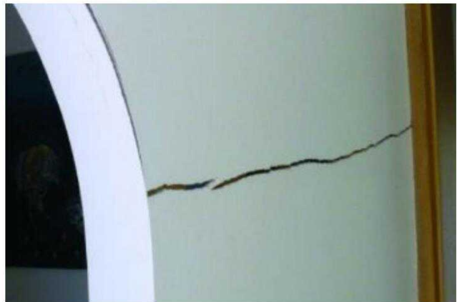
There are several doorways with cracks.
