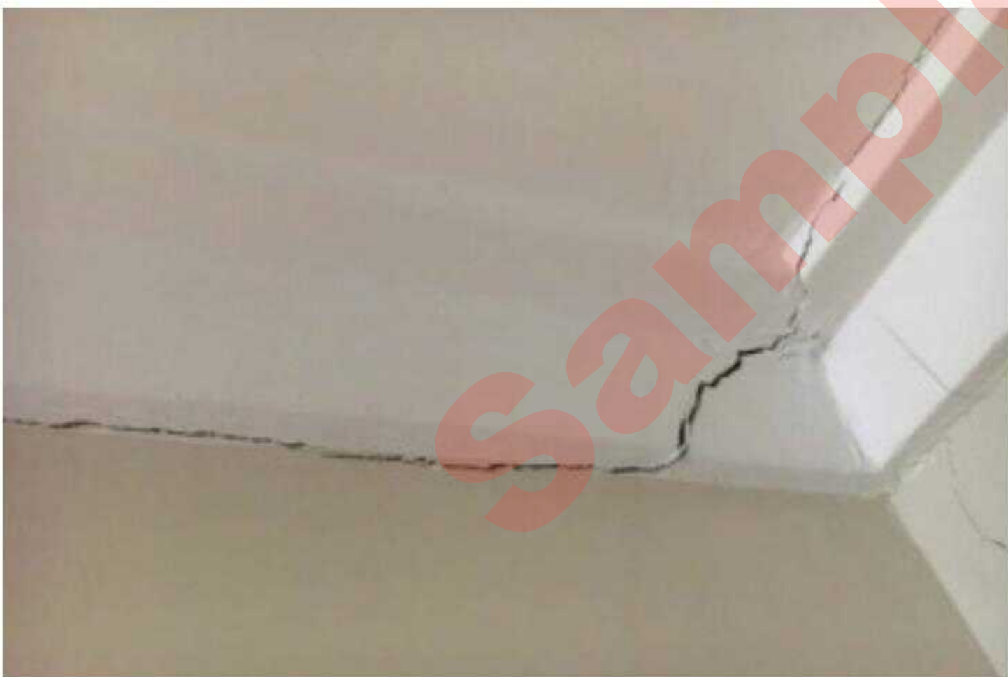
Crack in the ceiling and the crown molding in several areas.
