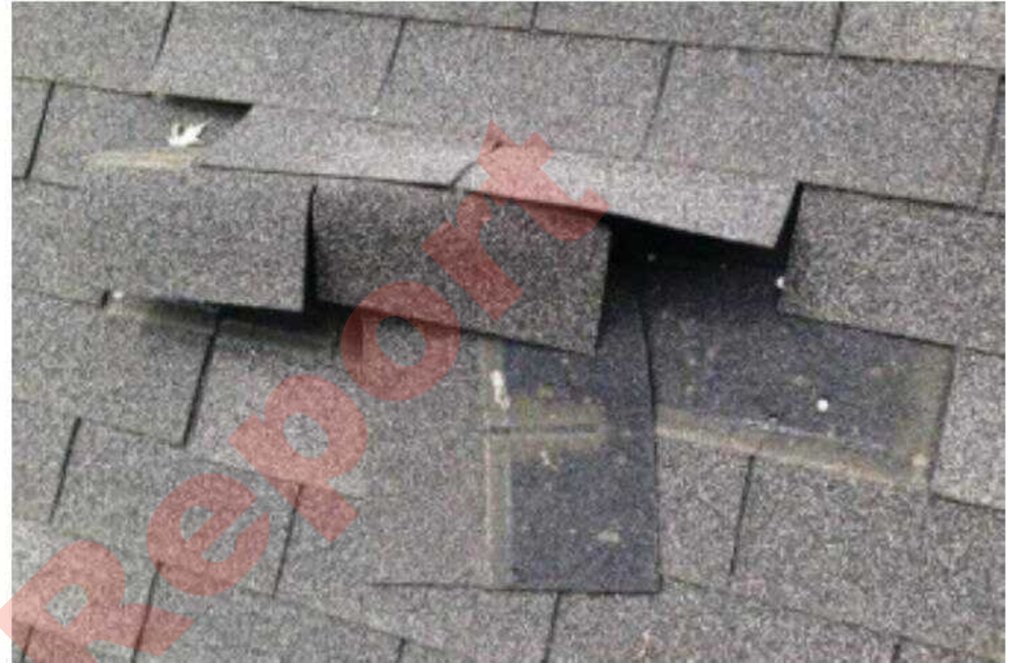
Another location where the tiles are pulled up and exposing the tar paper underneath.
