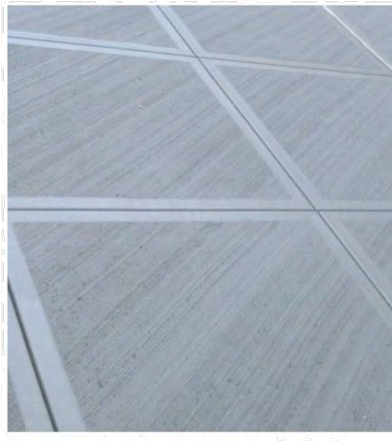
PATIO TOP AND STAIR TREAD FINISH broom-finish concrete with trowled control joints
