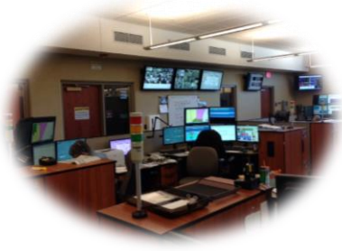
Public Safety Communication
