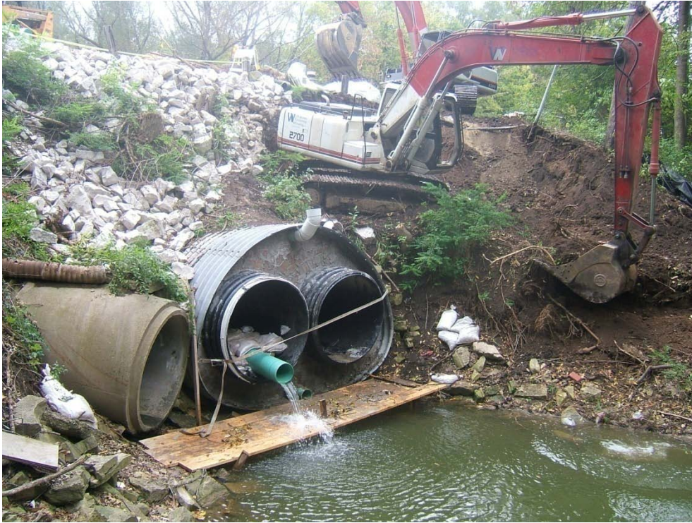
Figure 7.1 – The County Line Road culvert replacement project was completed with joint effort between the City of Mequon and the Village.
