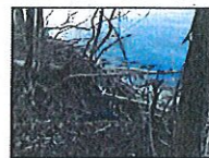
PHOTO 6: LOOKING EAST AT EROSION ABOVE EXISTING RIP RAP. FILL WITH STONE AS SHOWN ON CROSS SECTIONS.
