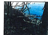
PHOTO 6: LOOKING EAST AT EROSION ABOVE EXISTING RIP RAP. FILL WITH STONE AS SHOWN ON CROSS SECTIONS.
