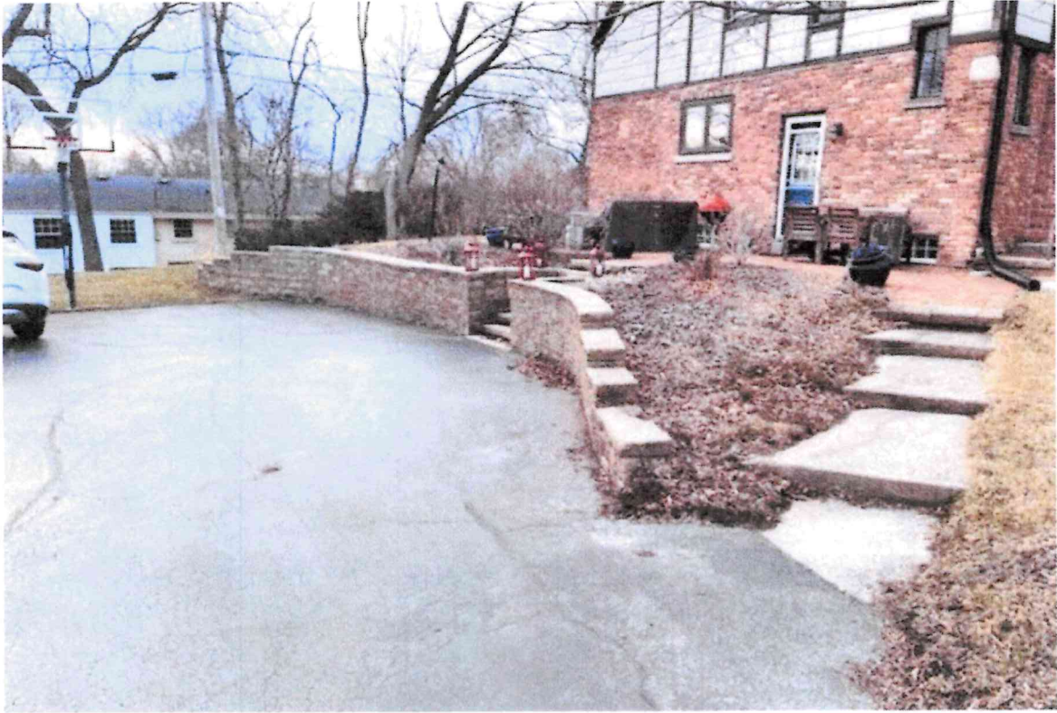
Existing failing retaining wall & Steps
