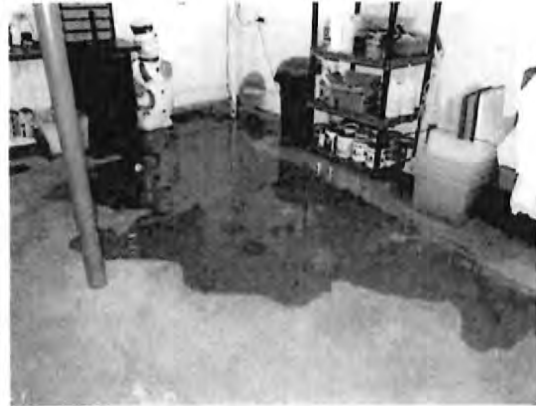
Standing Water Close-Up
