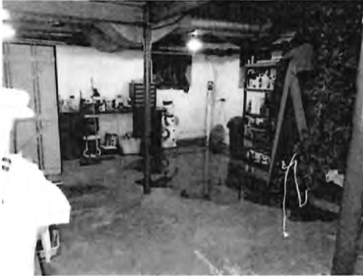
Basement with Standing Water
