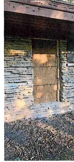
Emergency Door Opening 10/23
