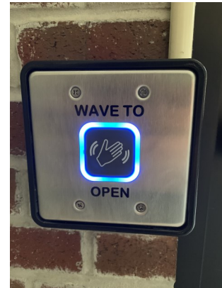
Touchless entries have been added to both the east and west entrances
