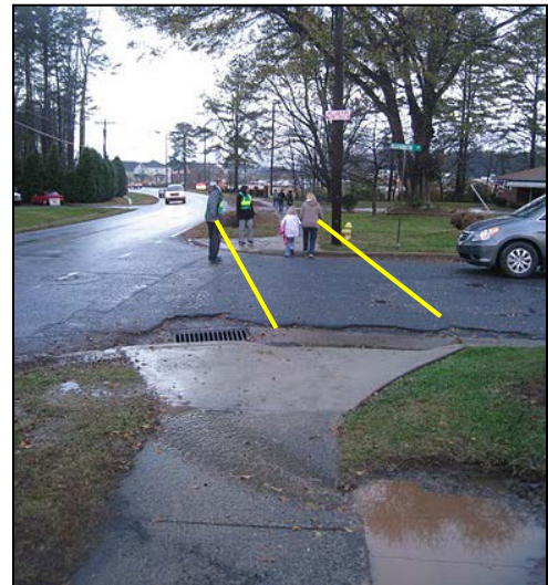
Figure 24 Elizabeth Street crossing looking west. Yellow lines highlight misalignment of curb ramps.
