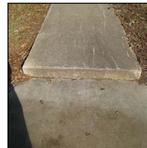
Figure 14 This pathway does not meet ADA guidelines.
