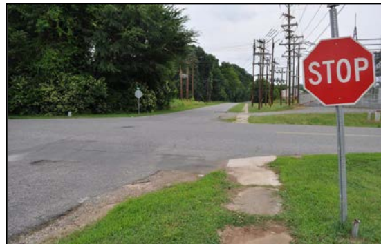
Figure 20 Intersection of Vine Street and Parkdale Drive lacks crosswalks and detectable warnings.
