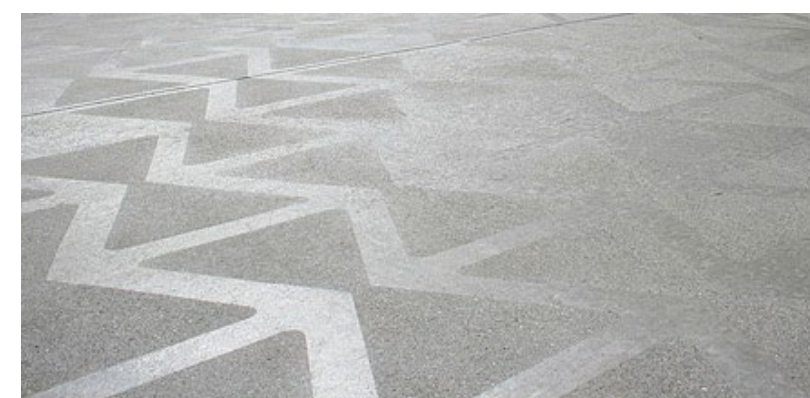
Poured in Place Decking- ADD Alternative Options (Bridge and Boardwalk) Not to Scale
