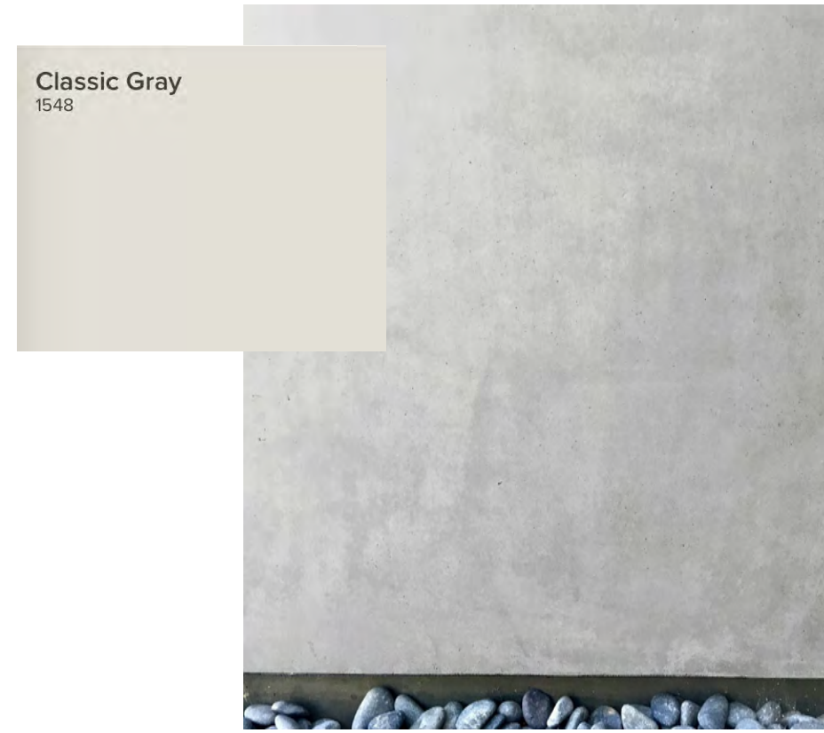
The existing stucco will be patched as needed and painted in a warm light gray color. Benjamin Moore's Classic Gray is a close Sample
