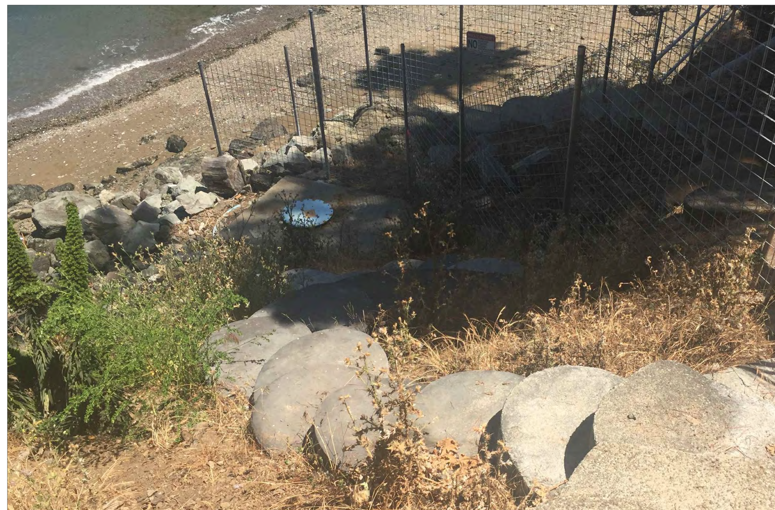
Looking toward shore line with new wire mesh fence and stepping stones in the foreground Sanitary sewer concrete tank and rip rap also shown
