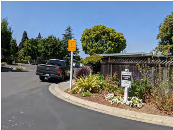
Intersections lack crosswalks and ADA-compliant ramps
