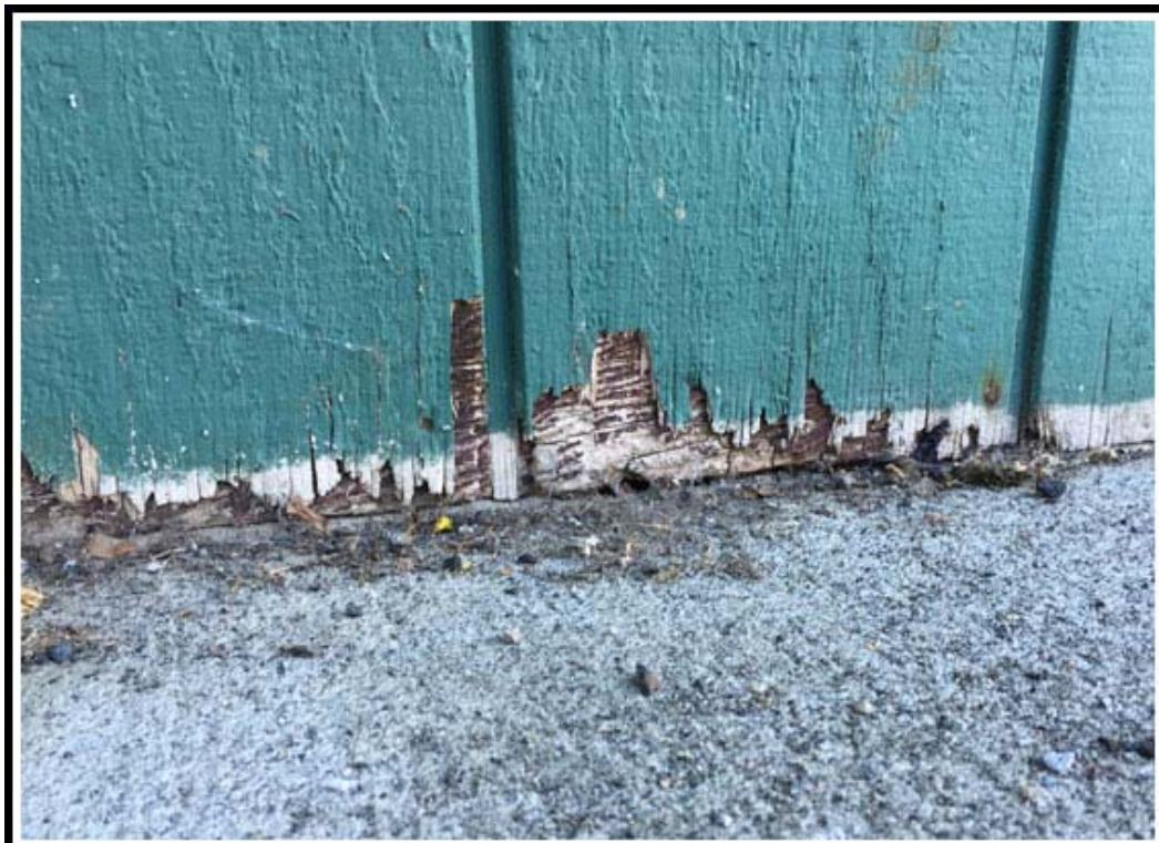
Photo 6 – Wood Siding on West Side of Building Extending to Top of Concrete
