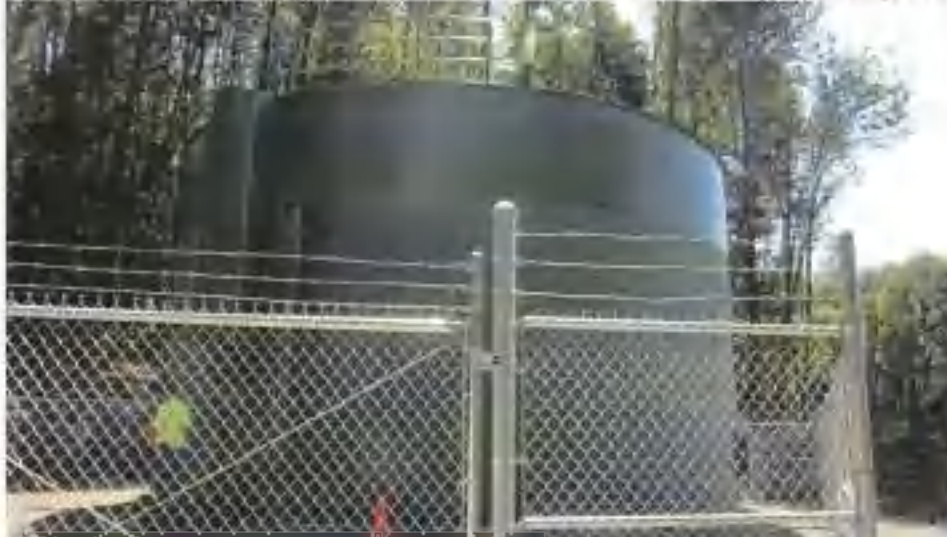
Spring Collection Tank (0.2M3): Overview of new Spring Tank.
