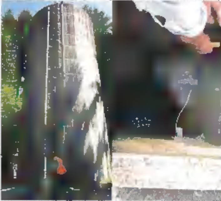
Existing 2.38K Reservoir: (L) Existing concrete tanks (see notes). (R) Existing overflow exits into catch basin with screen. Daylight with air gap and appropriate screening.
