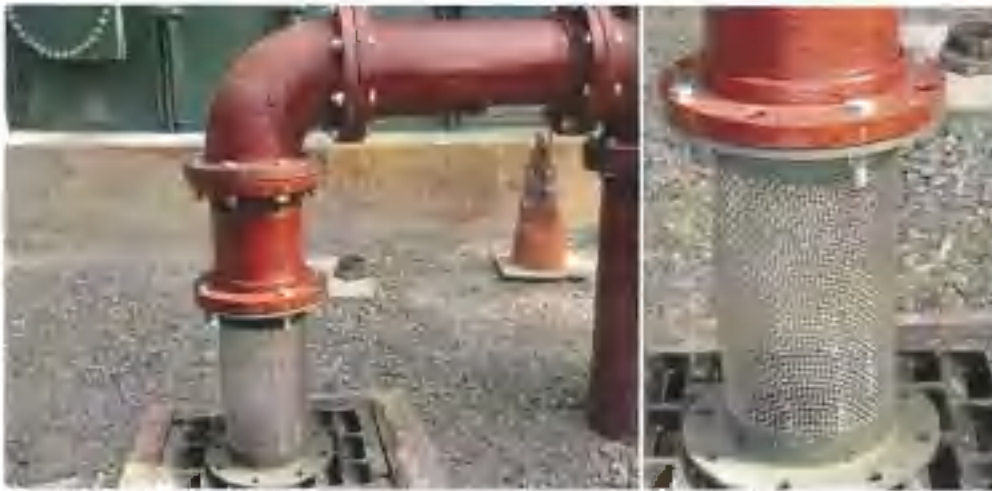
New 600k Reservoir: (L) Overview of overflow pipe daylighting above ground with air gap and screen. (R) Close up of vertical screen. Recommend installation of horizontal screen to prevent critters from crawling up pipe.
