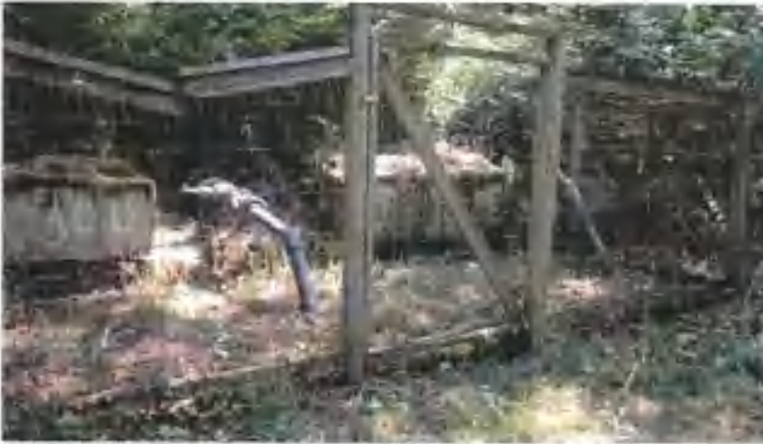
Horizontal Wellpoints: Overview of horizontal well points which also provide flow into system. Connect with transmission main which carries spring water to chlorination facility. May need to gather information on this source to determine if it is drawing water from same location as spring collection boxes; the Department will follow up with the City regarding this issue.
