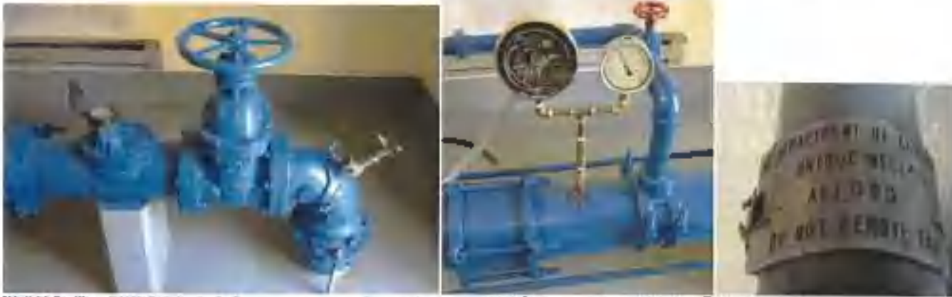
Well #1 Facility: (L) Well piping including source meter and raw water sample tap. (C) Mercury switch. (R) OUE Well identification tag.
