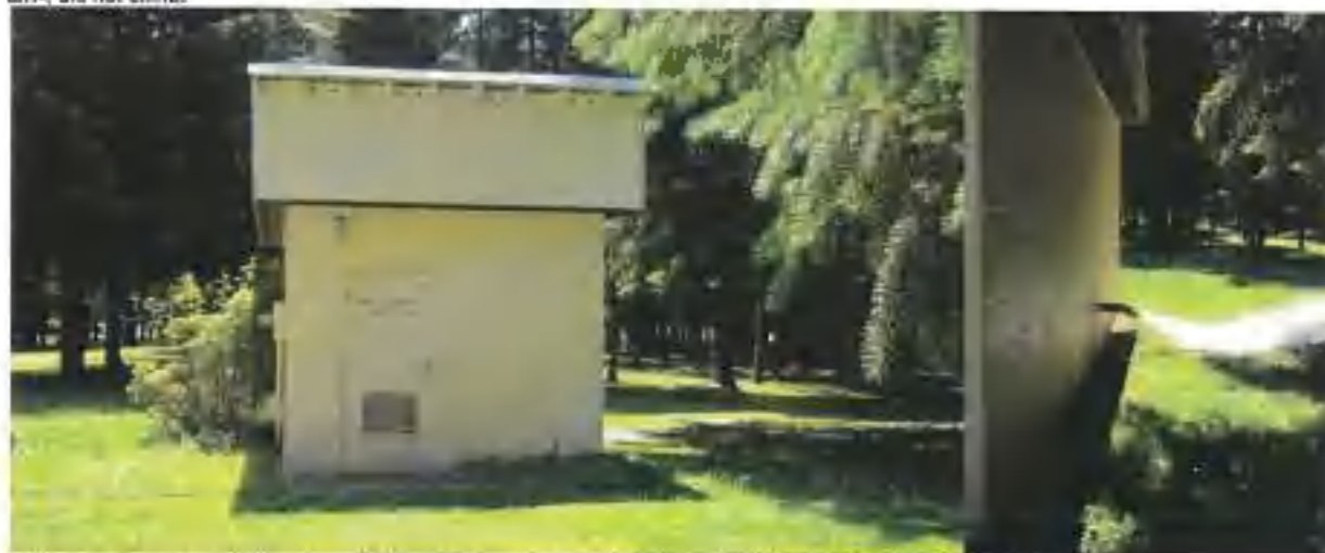
Well #1 Facility: (L) Overview of building located in park; not locked [check]. (R) Pump discharge; not screened.
