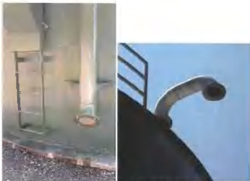
Spring Collection Tank (D.1 MG): (L) External overflow with air gap and horizontal screen. (R) Close up of reservoir vent with screen; one of several installed at top of tank; did not climb.
