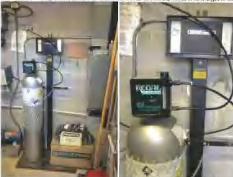
Spring Chlorination Equipment: (L) Chlorine gas cylinder for disinfection; typically use less than 1 lb per day; try to maintain residual 0.3 mg/L. (R) Regulator valve; manual controls. Measure chlorine residual at shop facility daily.
