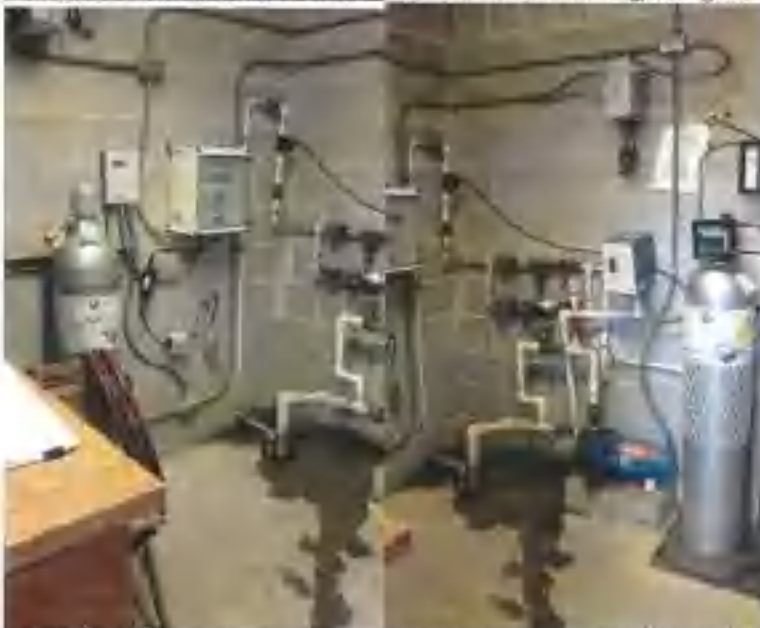
Spring Chlorination Equipment: (L) Interior piping/equipment showing chlorine analyser and controls for disinfection. (R) Pump and chlorine gas cylinder for disinfection. Pump draws stream of water from overflow vault, mixes chlorine gas in line.
