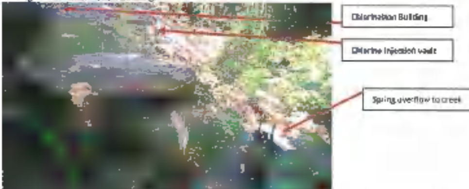
Spring Collection: (L) View of overflow vault, chlorination building would be on upper left. Overview to creek shown on right. Overflow vault has screen with vect. Locked access.
