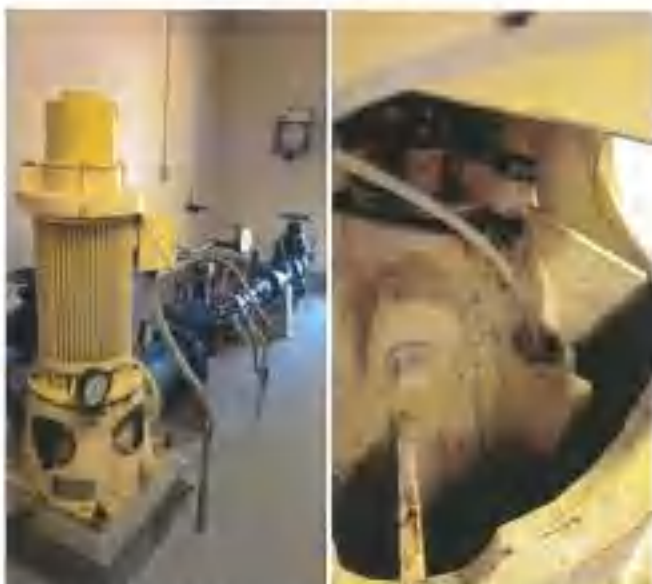
Well #1 Facility: (L) Overview of wellhead and piping. (R) Close up of sounding tube with latticed screen; fit with screened vane with gooseneck shape.
