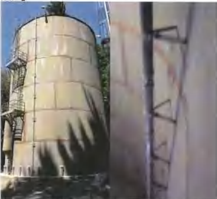
New 600K Reservoir: (L) Overview of new tank; not online during survey. (R) Picture of interior inlet pipe (or overflow) taken from manway at bottom of tank.
