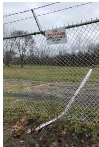
East side of Pitcher, vehicle hit fence.
