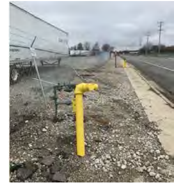
West side of Pitcher. Vehicle off road incident just missing water line.
