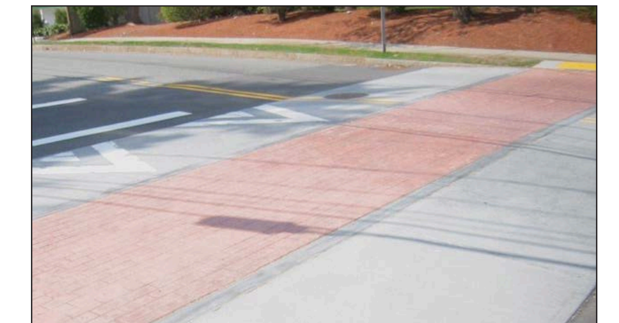
SPEED TABLE / RAISED CROSSING
