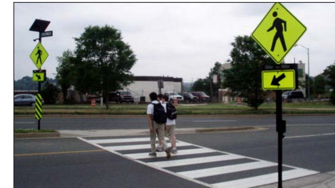
PEDESTRIAN CROSSING BEACONS
