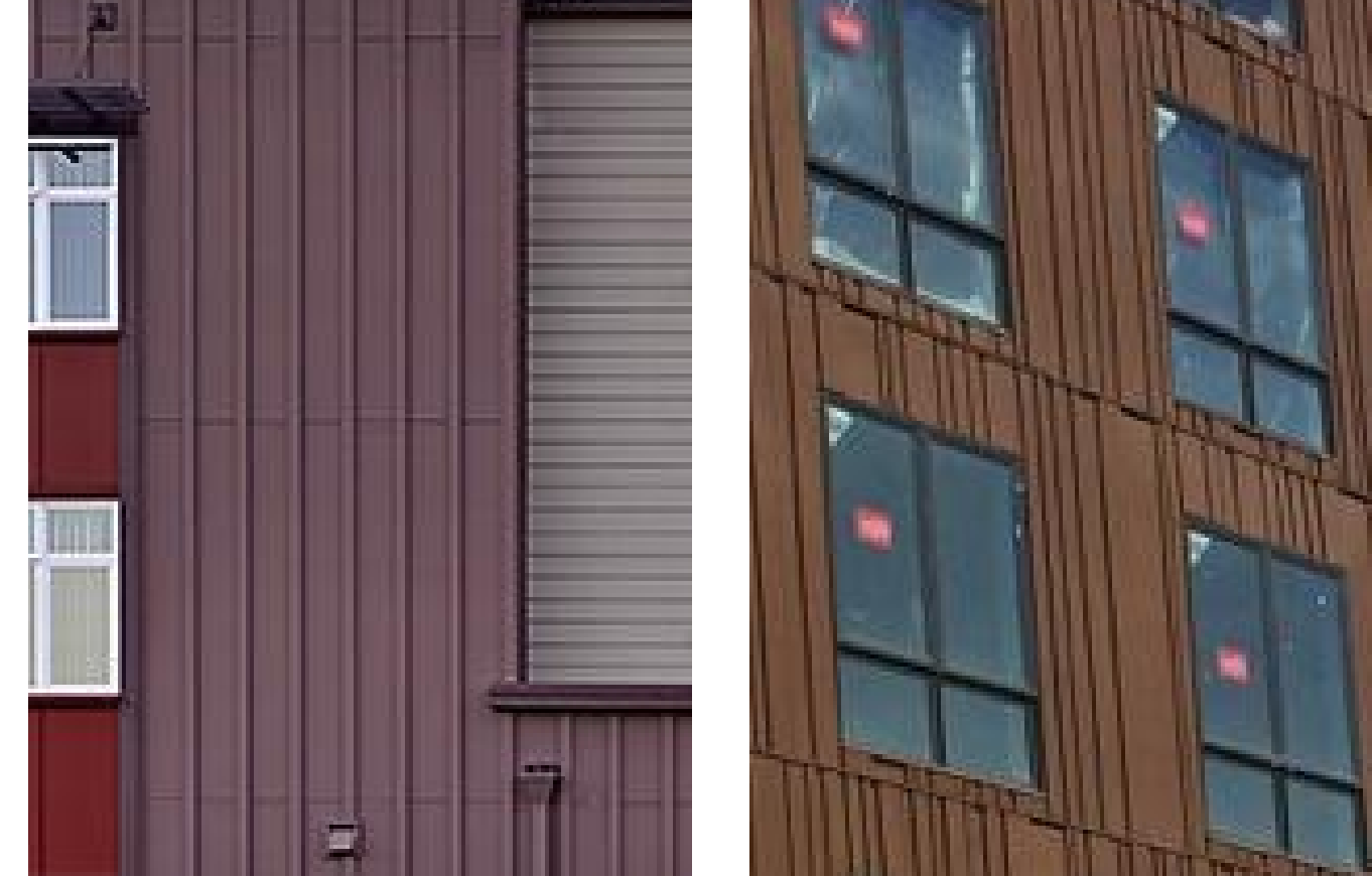
REGULARLY SPACED, TYP. RANDOMLY SPACED @ COMMON AREAS 6 A-5.2 FIBER CEMENT BOARD & BATTEN
