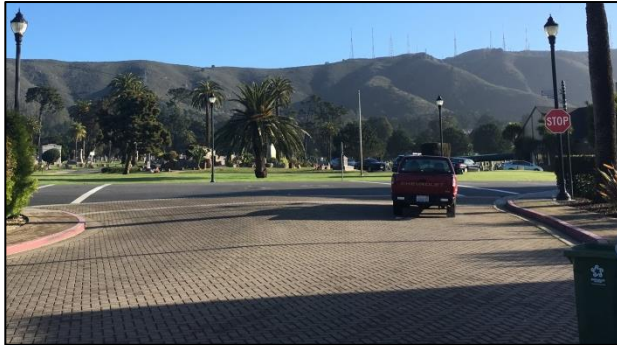
Lack of intersection markings (i)
