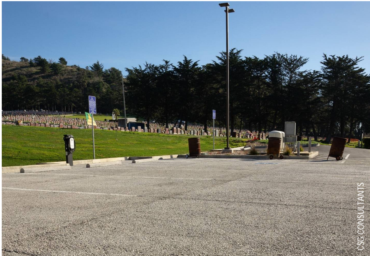
Porous pavement located at Golden Hills Memorial Park.
