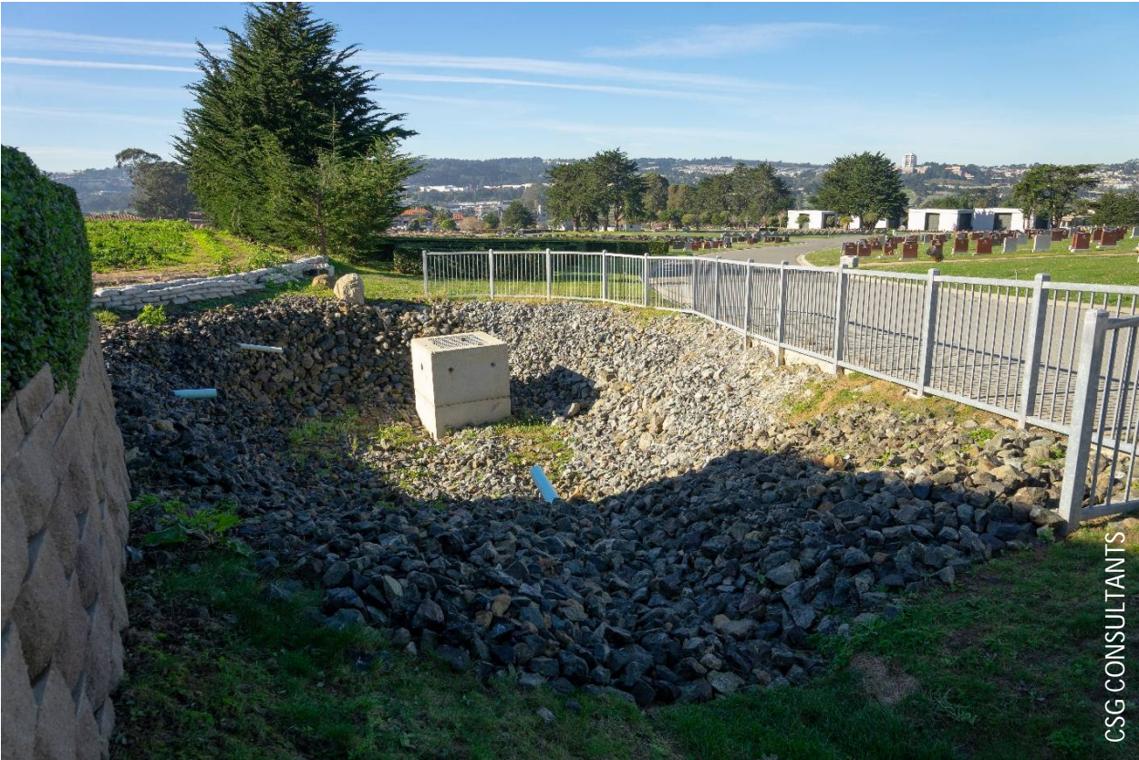
Detention system at Cypress Lawn Cemetery, which receives stormwater runoff from landscaping and bioretention areas.
